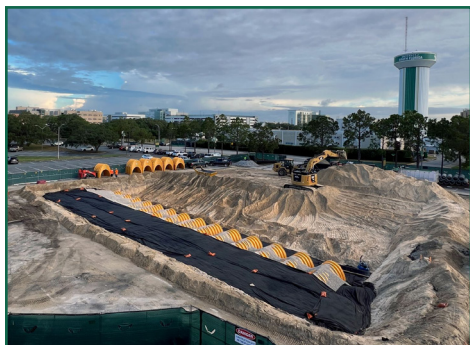
Stormwater mitigation initiative along Holly Drive aims to address frequent flooding issues and protect the university's central plant during periods of heavy rain.
