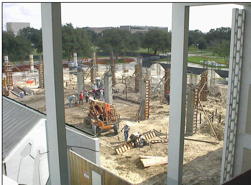
NES construction as seen from the third floor of the CHE building. The main support columns have been filled with concrete and their wooden casings are being removed. Taken September 10, 2003.
