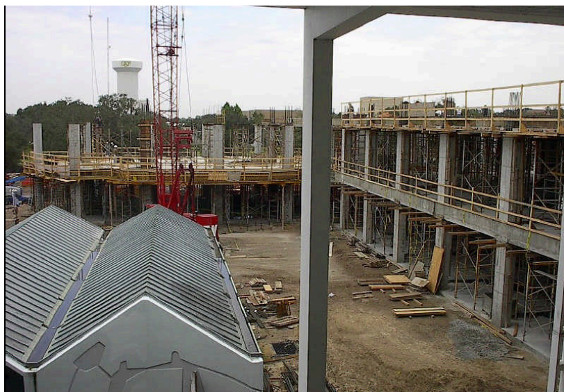
NES construction as seen from the third floor of CHE building. Taken October 20, 2003
