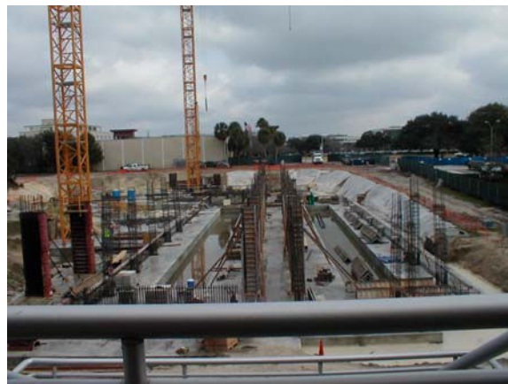
Future Seven-story Interdisciplinary Science Teaching & Research Facility (ISA). Picture taken in January from third floor of Chemistry; Administration Building is in background.
